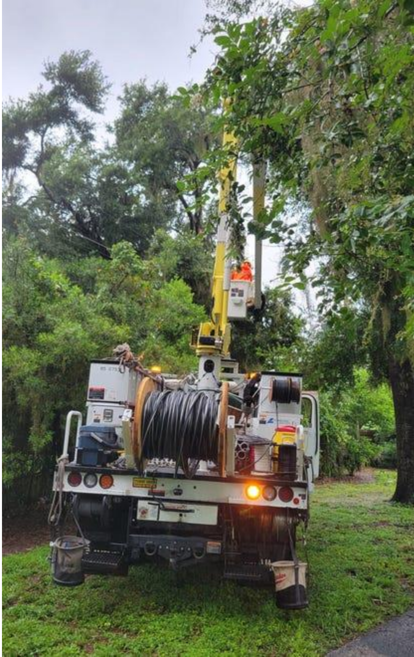
A crew from Lakeland Electric works to remove fallen branches from power lines along the south edge of Dobbins Park on Monday morning. Power was out to some houses in the area for about five hours before being restored in mid-morning.
