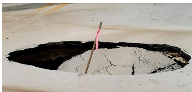
Figure IV.9: Sinkhole/Depression middle of Kathleen Road September 2012; Source: The Ledger
