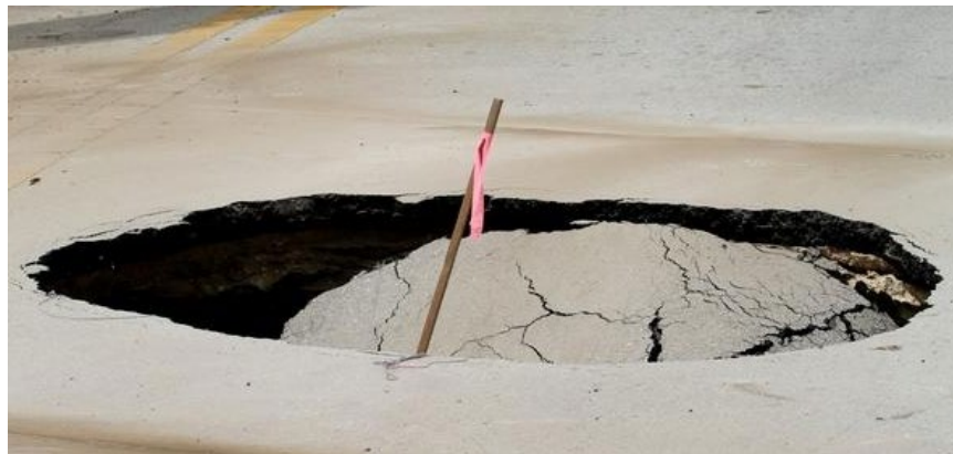
Figure V.20: Sinkhole in Kathleen Road from collapsed pipe
