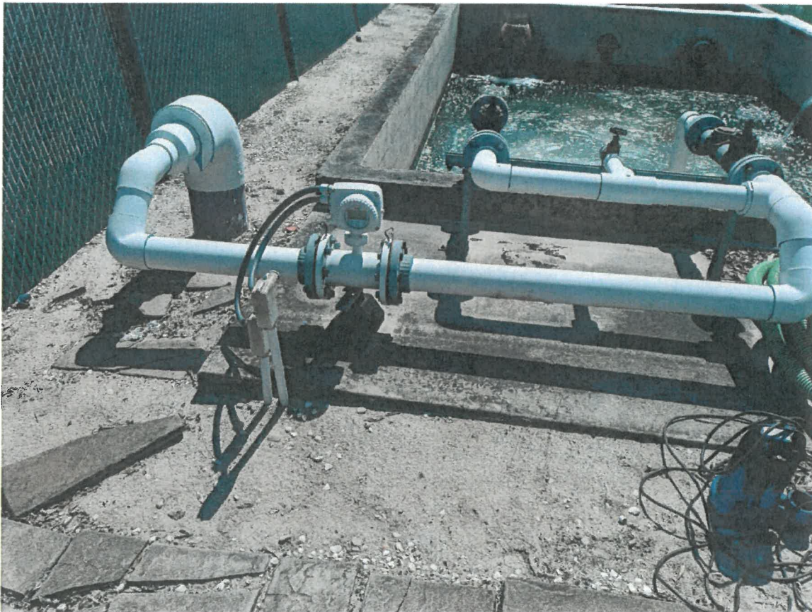
EFFLUENT DOSING TANK AND FLOW METER
