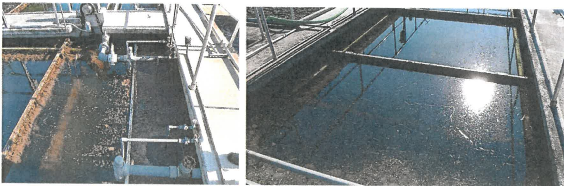
STILLING WELL AND CLARIFIER SURFACE
