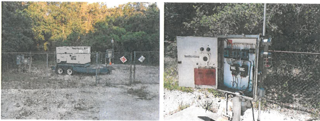
LIFT STATION #1 AND CONTROL PANEL
