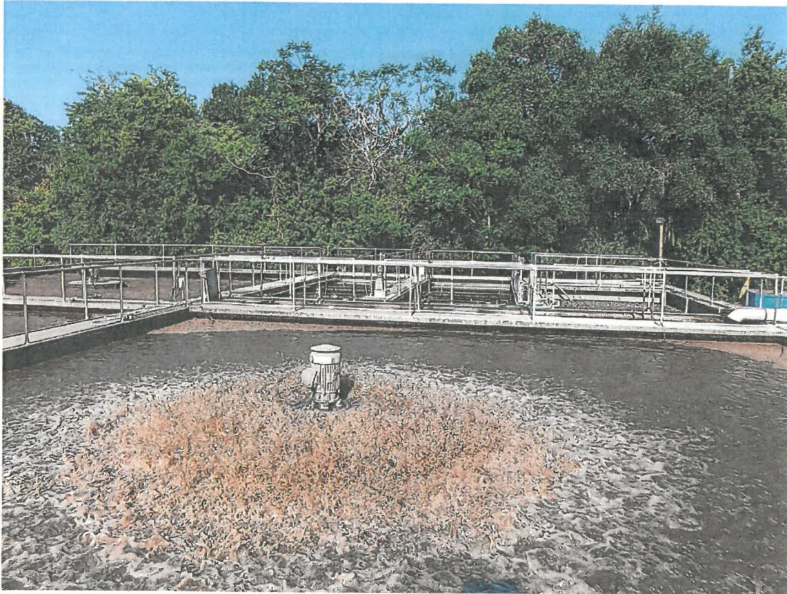
AERATION TANK MECHANICAL MIXER
